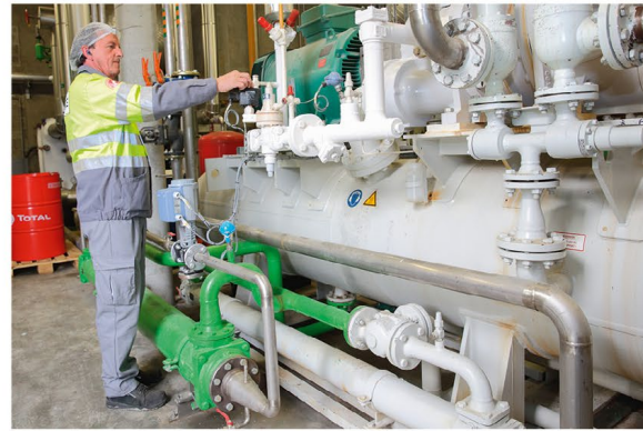
Heat recovery system
