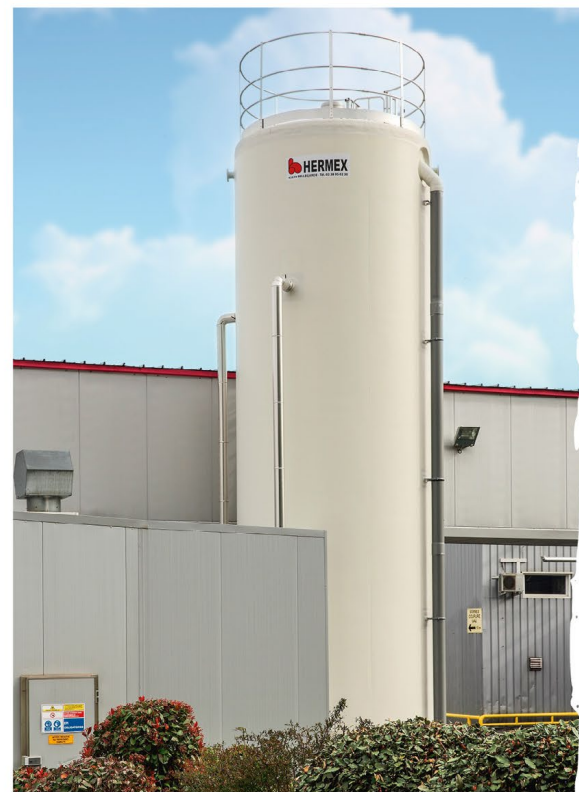
Heat recovery tower
